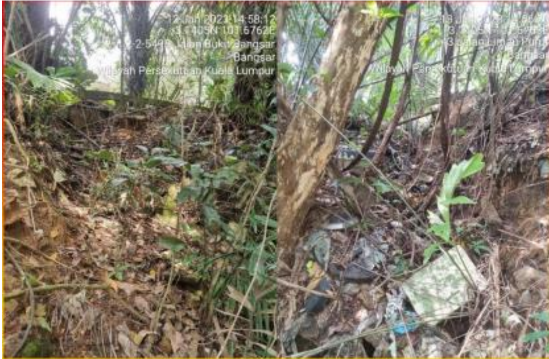
Plate 2.3: The damaged drainage belongs to one of the buildings that pours its surface water runoff directly into the steep terrain of Pulai Trail Urban Community Forest. The formed gully erosion is filled with plant debris and waste.
