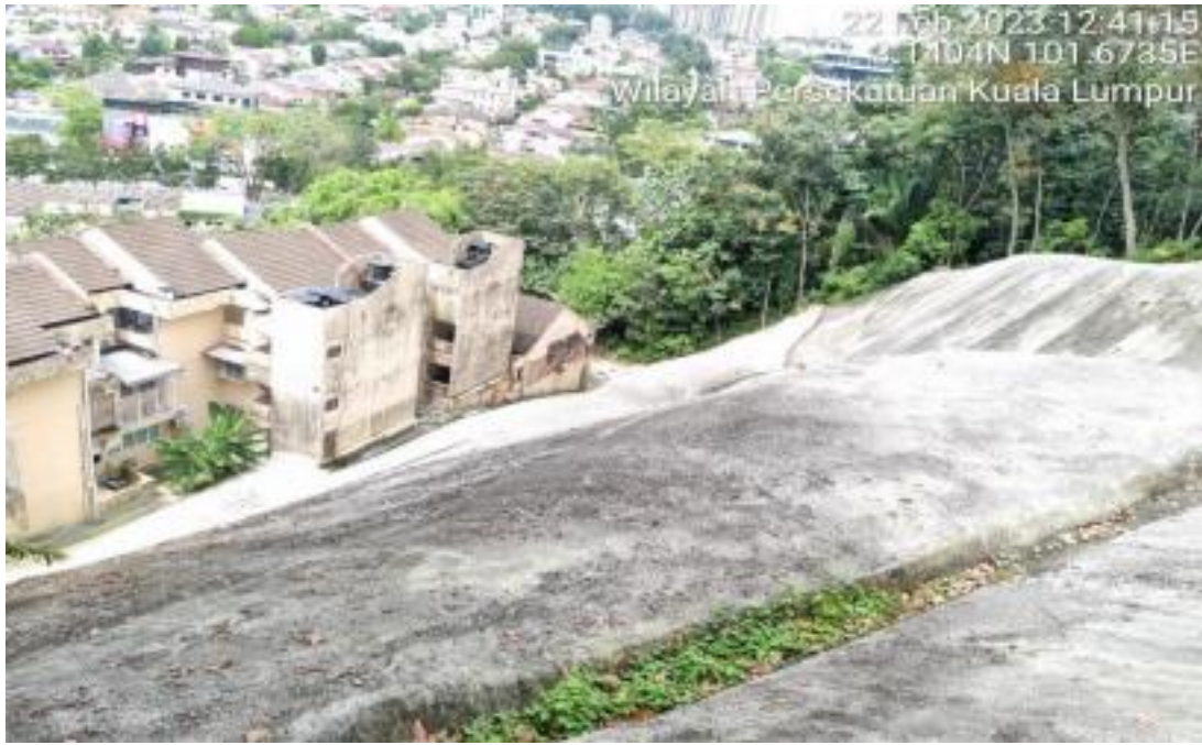
Plate 2.4: Concrete retention wall is used to replace the natural regrowth on the slope. The slope is concreted to prevent surface erosion that may lead to landslide. The slope was behind the Club Veteran Komando Malaysia.
